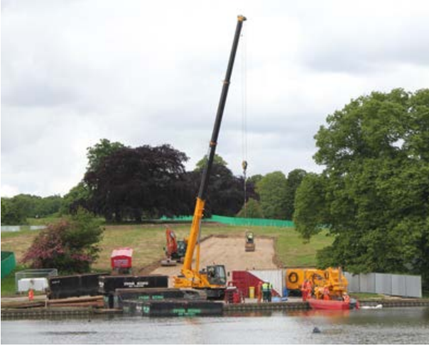
Picture 1 -Sheet metal piling to create temporary dam at Model Boating Pond.
